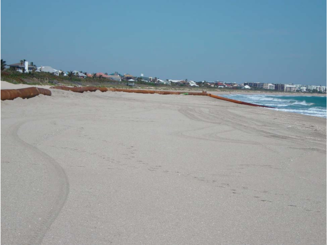
Figure 5. Discharge Pipe Beach Landing. The submerged pipeline from the dredge extends up the beach and is connected to pipe sections that extend down the beach as construction progresses. The beach shown in this photo was constructed from the dredge material.
