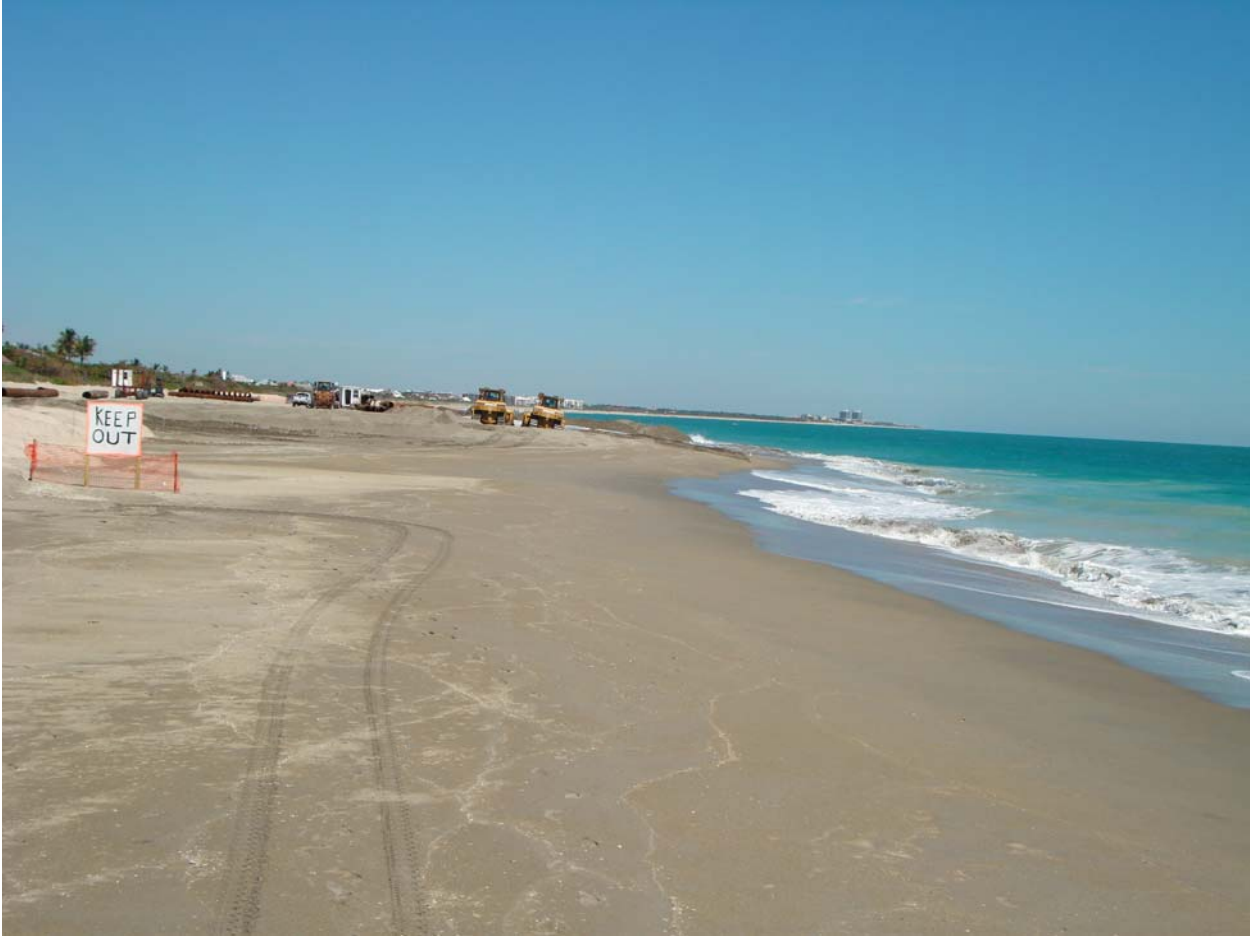
Figure 3. Beach Discharge Location. Note security fencing in foreground. Equipment and pipe storage and staging is present. Discharge occurs in the vicinity of the two bulldozers.
