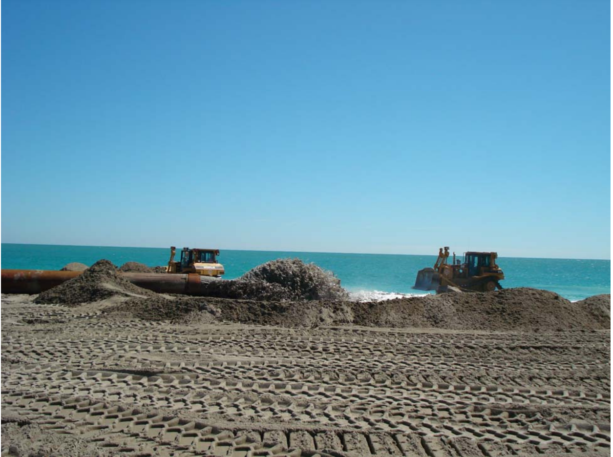
Figure 4. Close-up of pipe discharge. The two bulldozers are required to grade the placed material, direct the discharge, and maintain the construction dikes. These operations occur 24 hours per day, 7 days per week.
