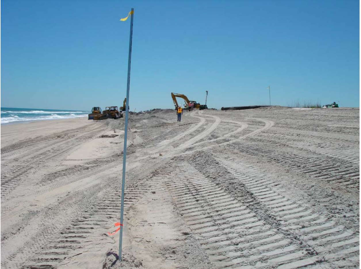
Figure 7. Finished and Graded Beach Face. Note the construction/discharge operation in the background and the grade stake in the foreground.
