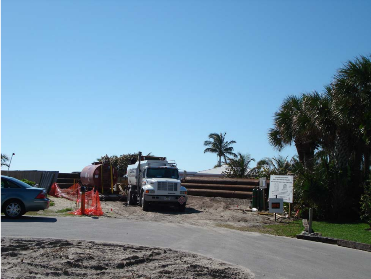
Figure 1. Upland Beach Access/Staging Area. This site is representative of the staging area required at the beach access site. Fuel delivery activities are occurring in the photo. Pipe sections are also visible in the background.
